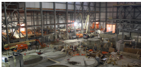
Gold recovery area in plant building
