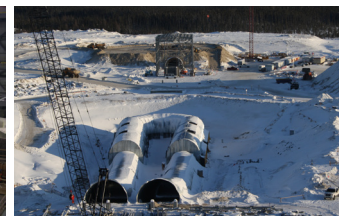
Primary crusher and stockpile reclaim
